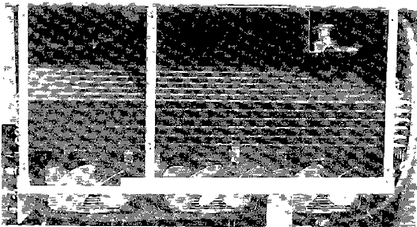
Air cooled condenser
